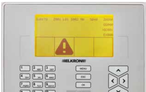
YELLOW System failure/malfunction
